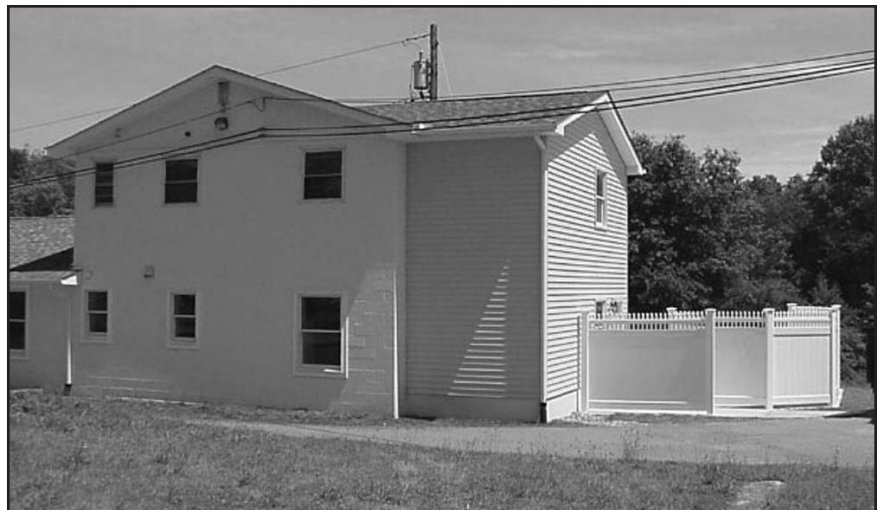
Renovation of the Steppingstones residence on the grounds of the agency’s headquarters is underway for the relocation of the agency’s Respite house.
